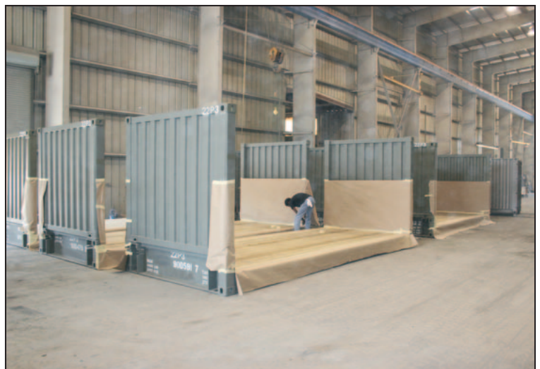
Pressure treated wood plank floors being prepped for Polyurea application. See back for finished application.
